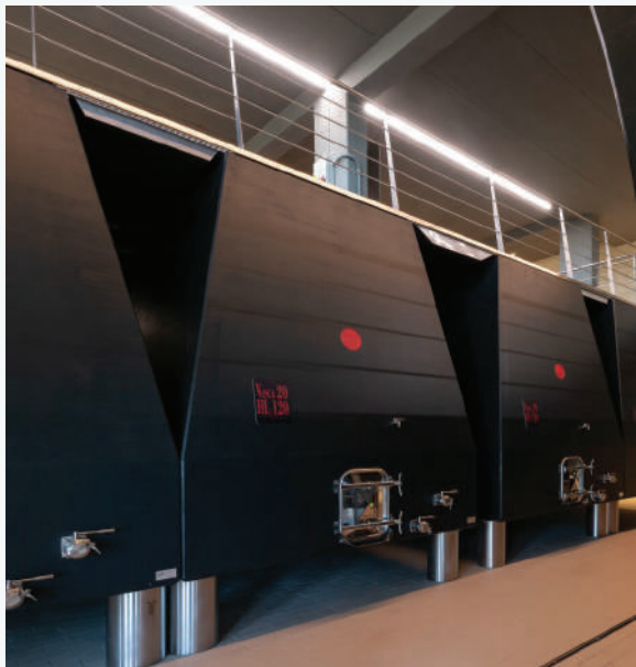
Line of Tronco tanks.
